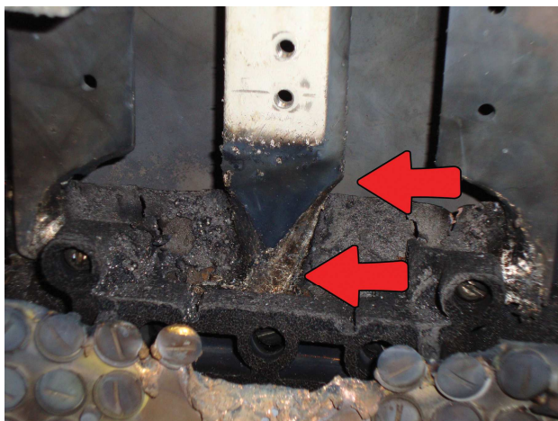
Fig. 4. Erosion of aluminum busbars from panel arc fault.
